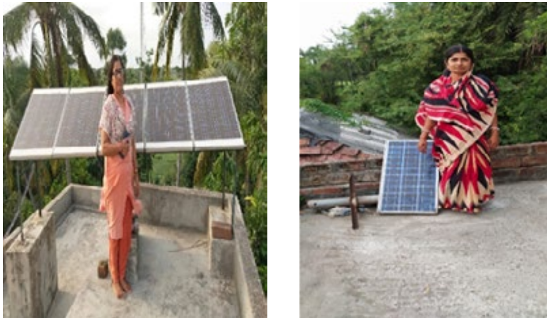
Women in front of unused PV solar panels in need of repair and maintenance in Sagar
